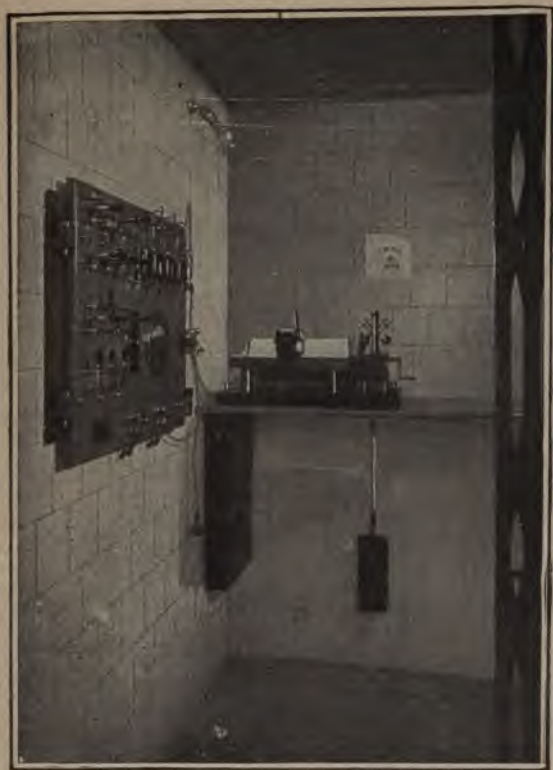
View in outer passage of Clockroom showing chronograph and switch board.
